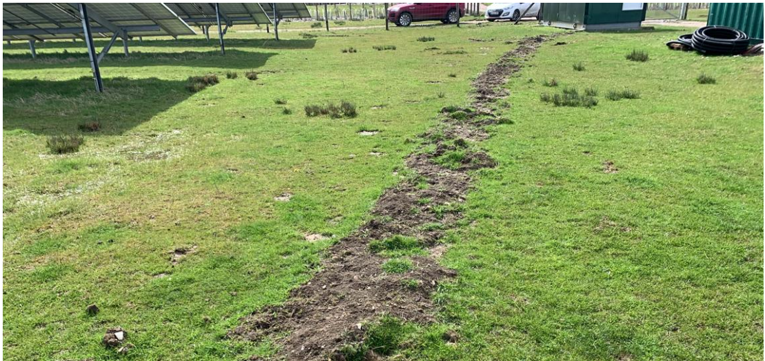
Photo 15.22: Trench During Wet Period
